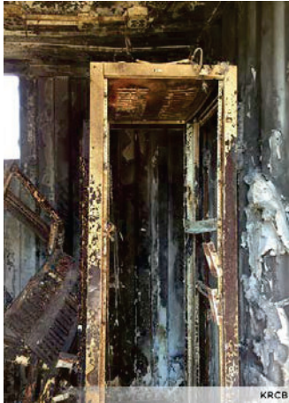
Above: The interior of KRCB-FM's transmitter building after a fire in October 2019.
